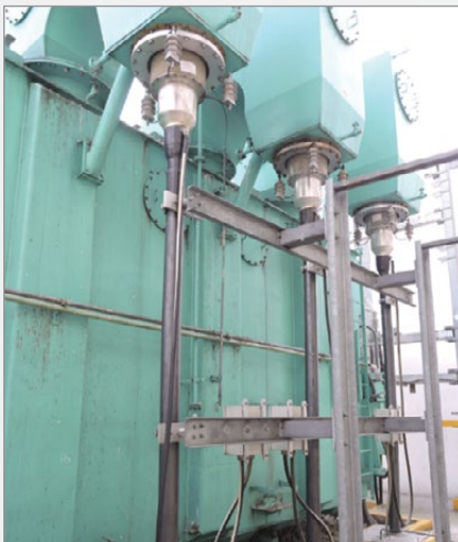
Terminations of a 230 kV short cable system
