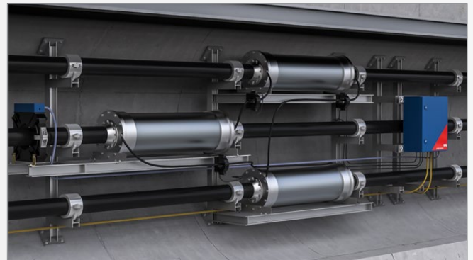
PD monitoring at the cross-bonded joints of a tunnel cable system
