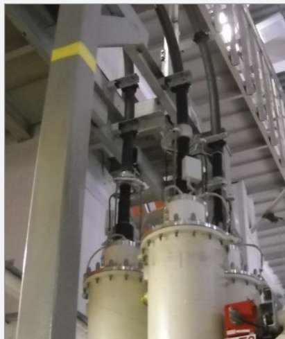
Terminations of a 380 kV buried cable system
