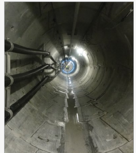
Joints of a 380 kV tunnel cable system
