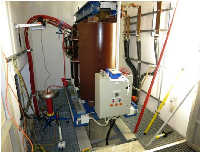
Figure 9. PD measurement setup on a 20 kV / 2 MVA cast resin transformer
