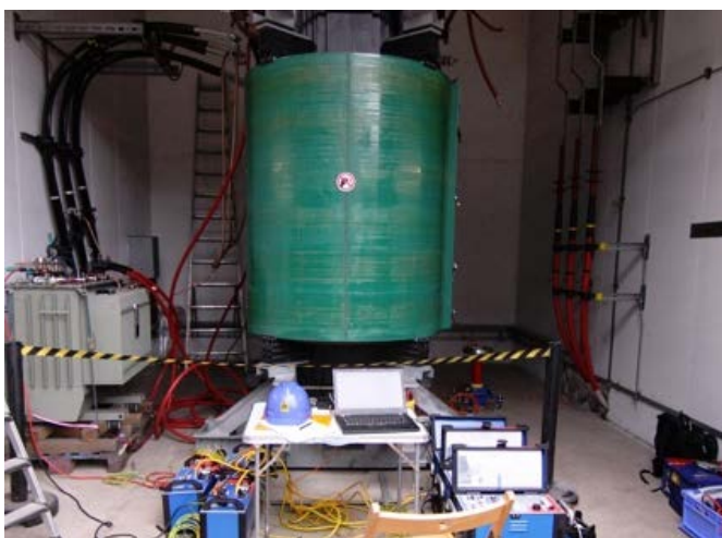
Figure 11. PD measurement on a 17 MVA cast resin transformer using three CPC 100
