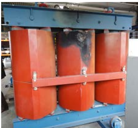
Figure 7. Breakdown fault on cast resin transformer
