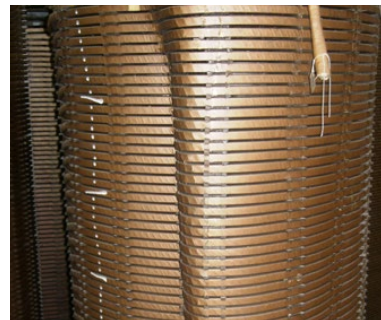
Buckling of winding
