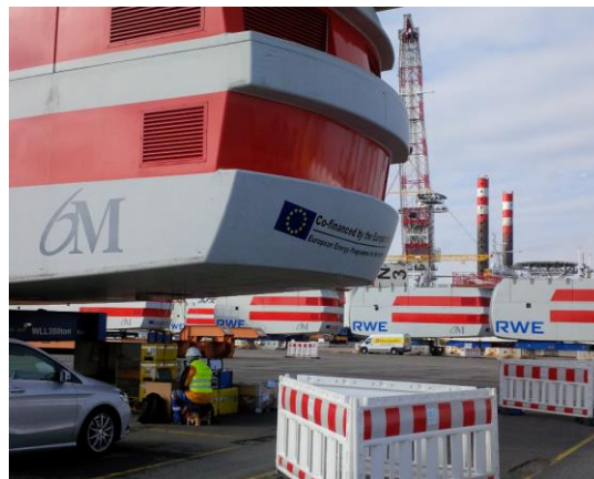
Fig. 8: On-site PD-test to verify the functionality of the CPC-source on an installed transformer
