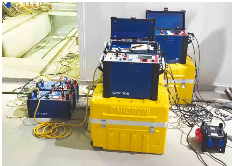
Three CPC 100 units with CPC Sync and three matching transformers were used for excitation of the dry type transformers.
